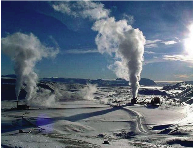
7. The Krafla is a geothermal power station located in Iceland. (Credit: Wikipedia Commons/Ásgeir Eggertsson)
